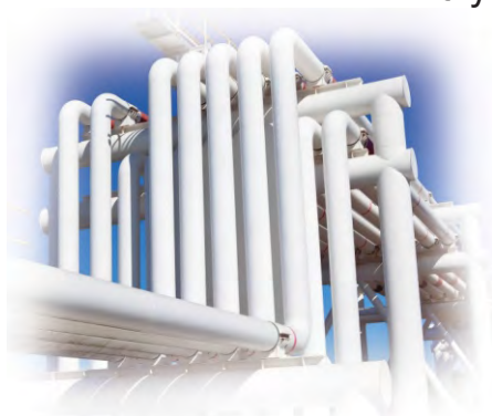
Industrial Gases Pipeline
